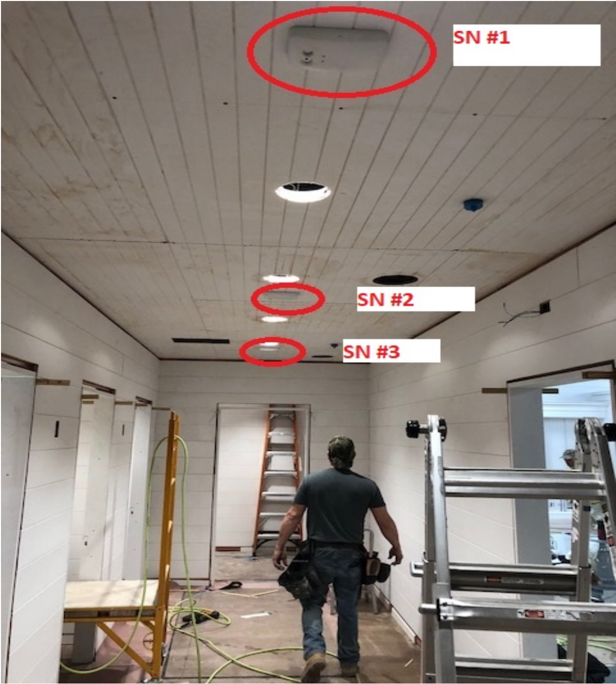
Sensors installed equally spaced
